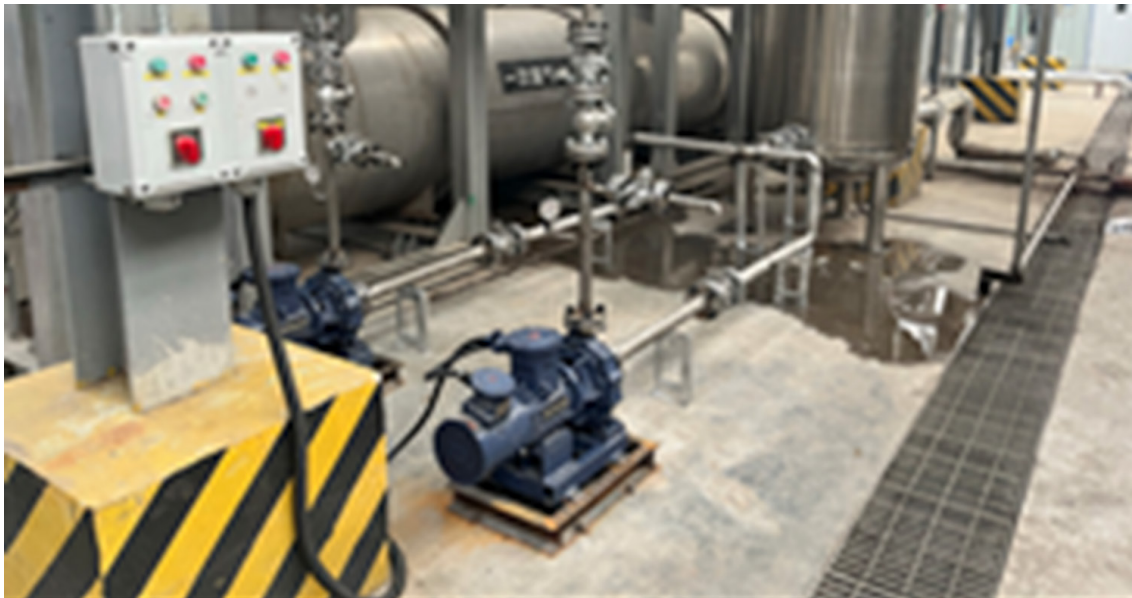
Sichuan AET Steam Condensate Recovery
